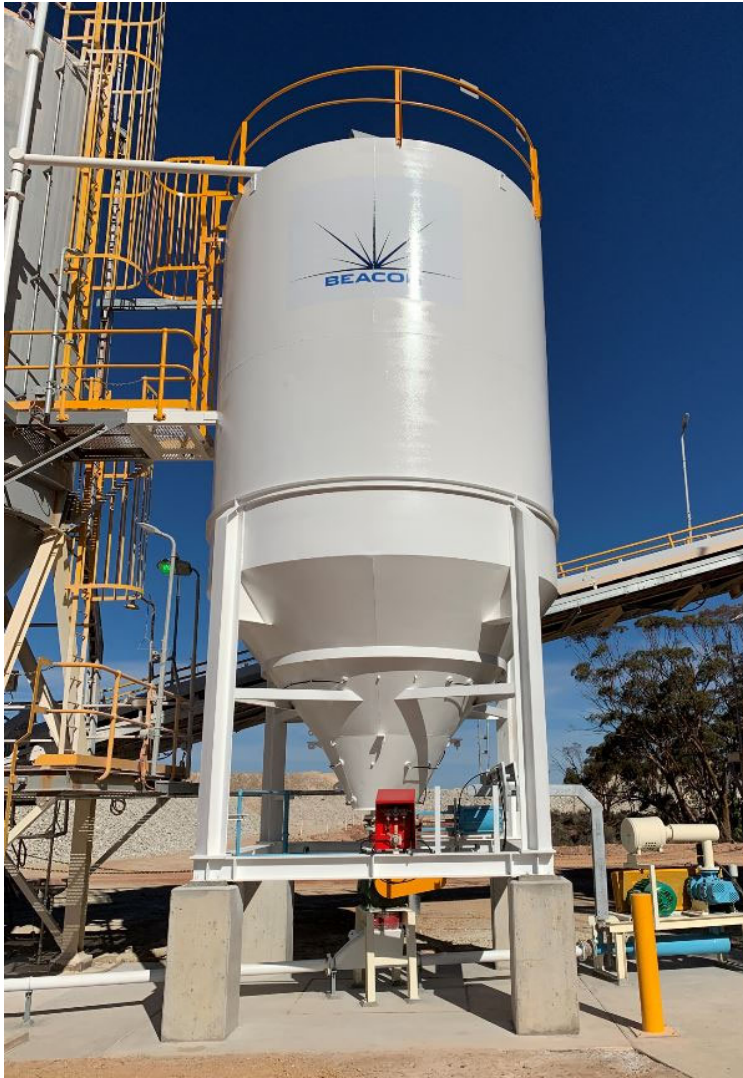
Figure 3: Jaurdi Gold Project – Additional Lime Silo
